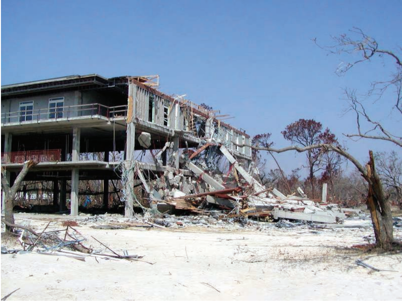
Figure 2-28 Concrete frame of three-story apartment building that partially collapsed due to failure of the post-tensioned flat slab in the bay closest to the Gulf of Mexico (Hurricane Katrina, 2005).
