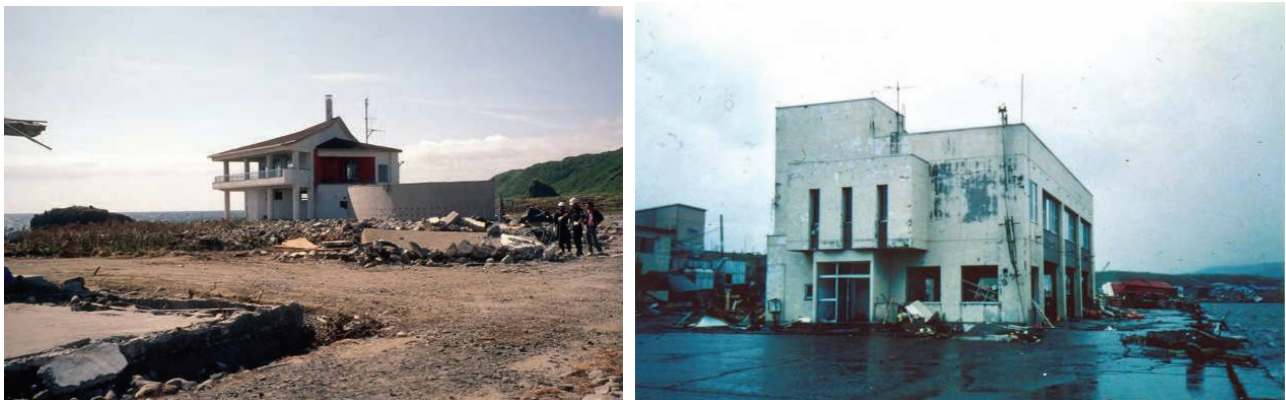
Figure 2-13 Examples of reinforced concrete structures that survived the 1993 Okushiri Tsunami: vista house at Cape Inaho (left); and fish market in Aonae (right) (Photo courtesy N. Shuto).
