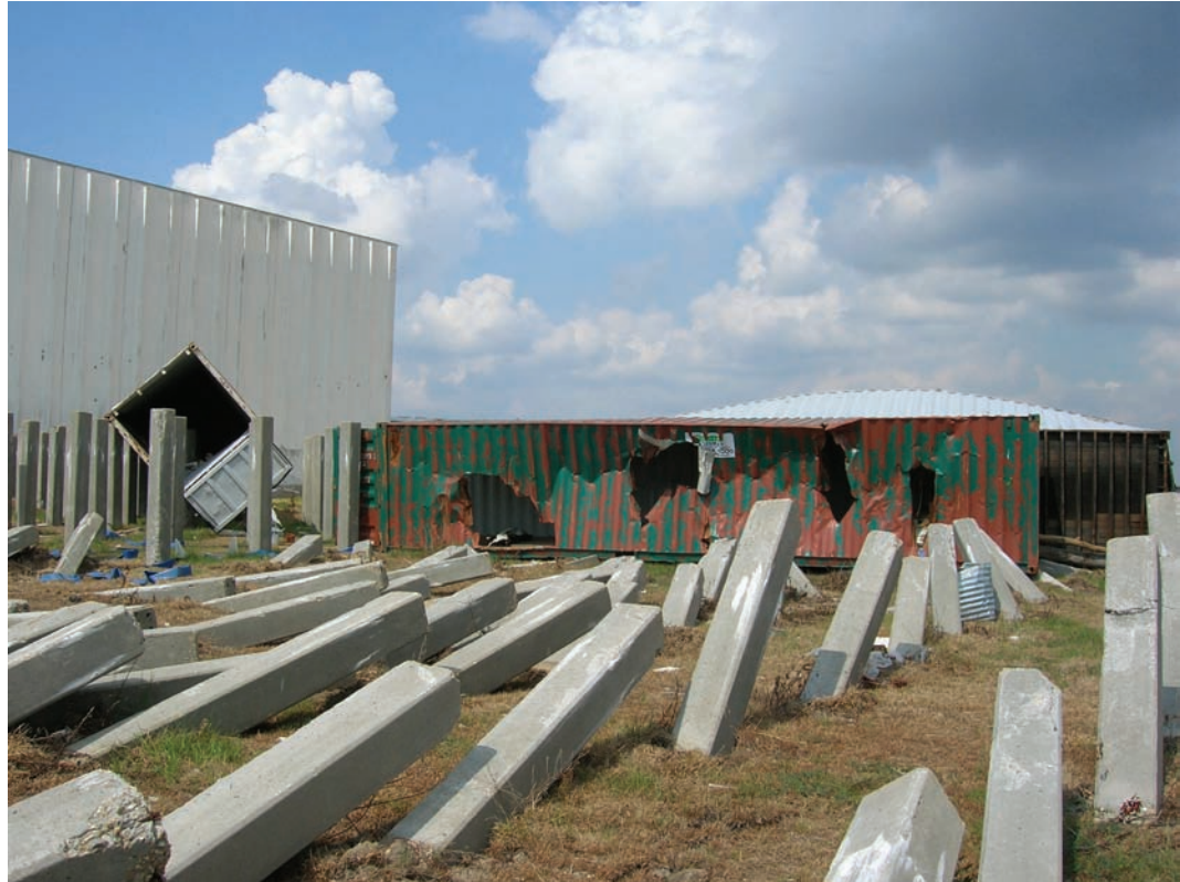
Figure 2-26 Failure of prestressed piles due to damming effect of shipping container (Hurricane Katrina, 2005).
