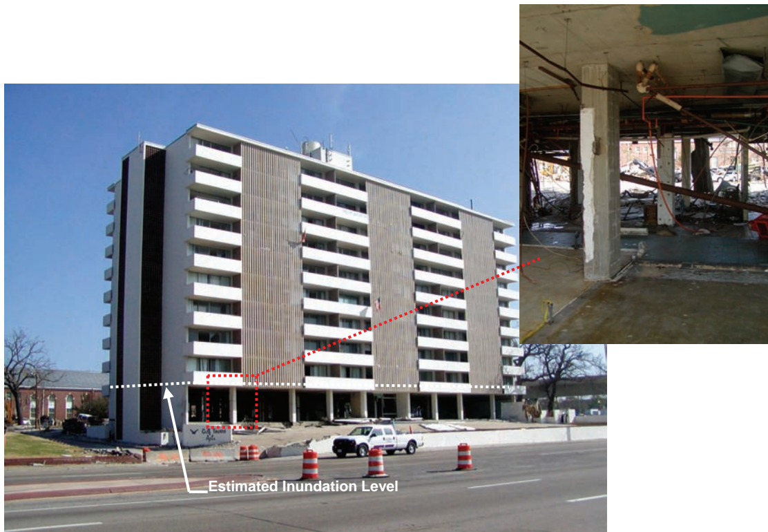
Figure 2-22 Gulf Tower Apartment building suffered substantial non-structural damage at the ground floor level, but remained structurally sound (Hurricane Katrina, 2005).
