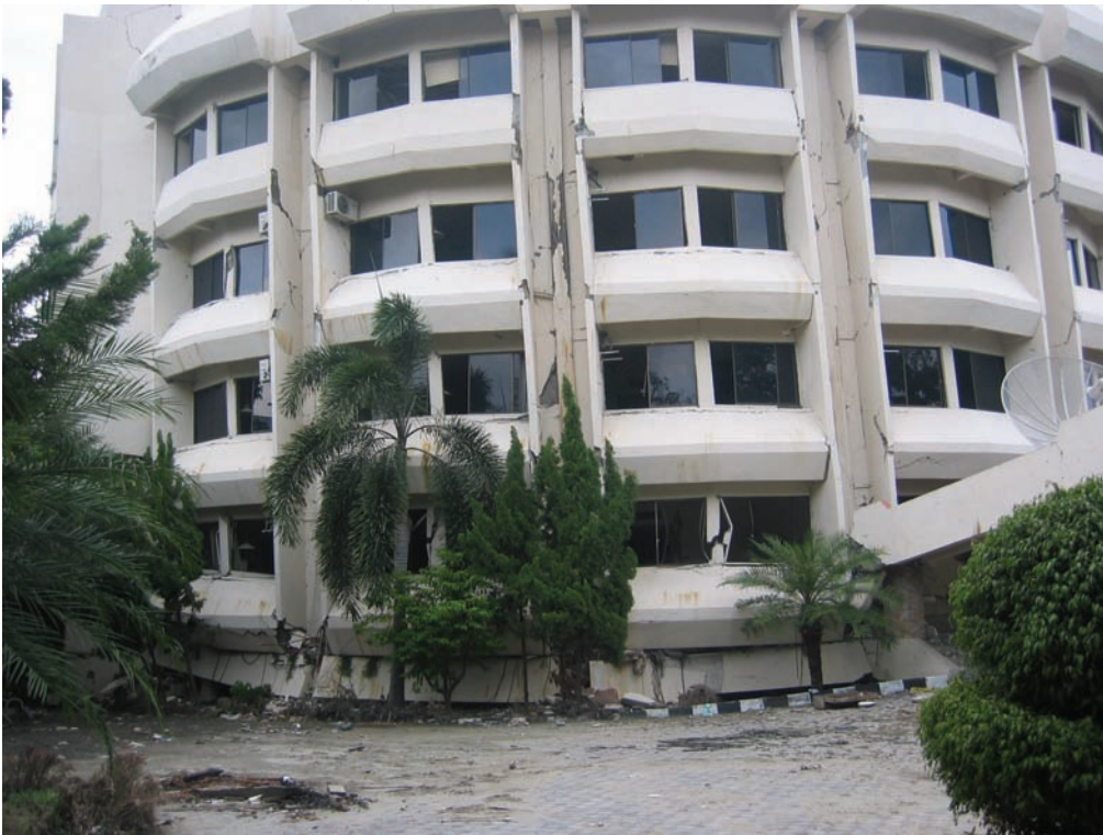
(b) Soft story failure
