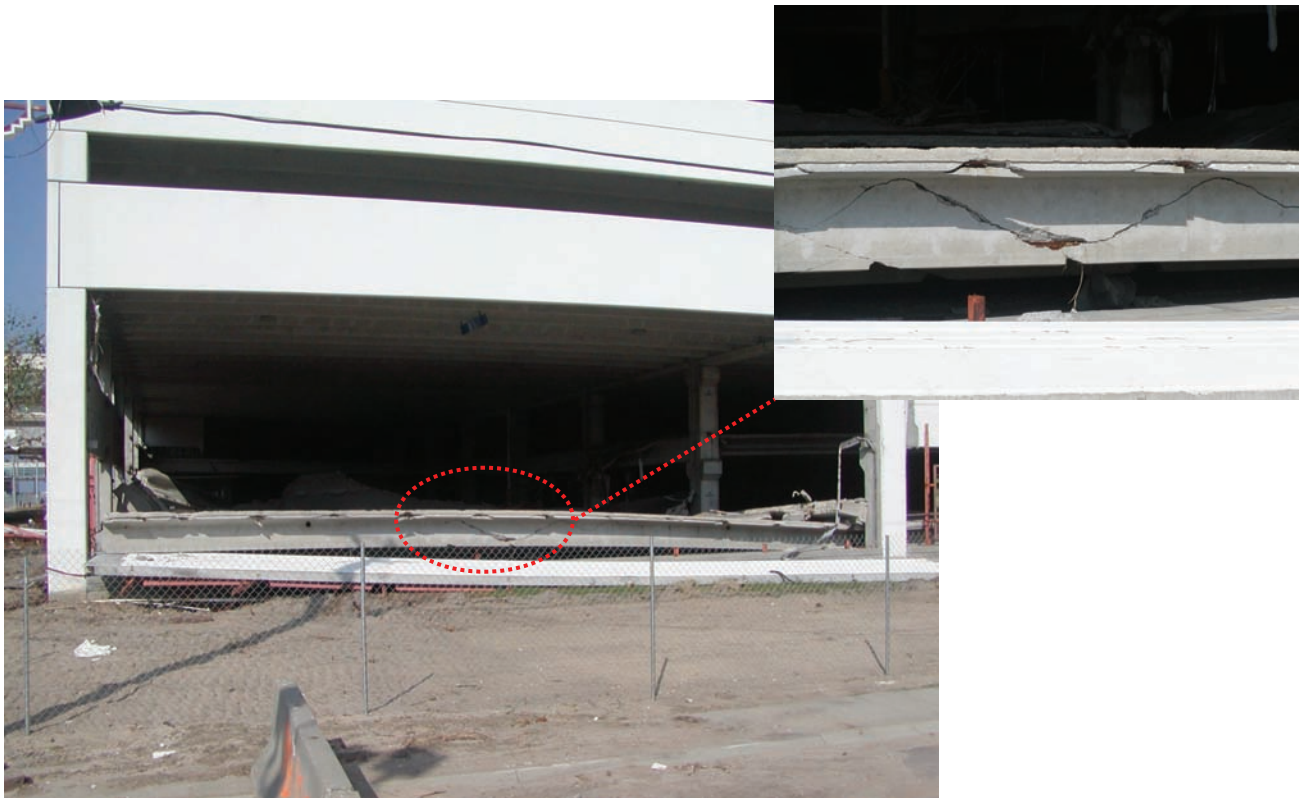
Figure 2-27 Negative bending failure of a prestressed double-tee floor system due to uplift forces (Hurricane Katrina, 2005).
