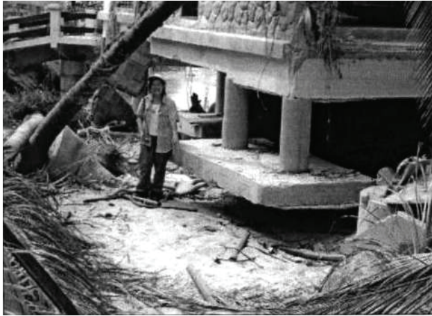
Figure 2-19 Scour around shallow spread footing in Khao Lak area (Dalrymple and Kriebel, 2005).
