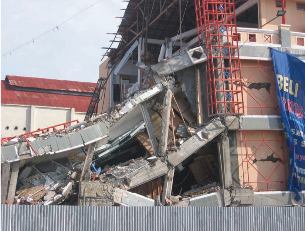
(a) Beam-column connection failures
