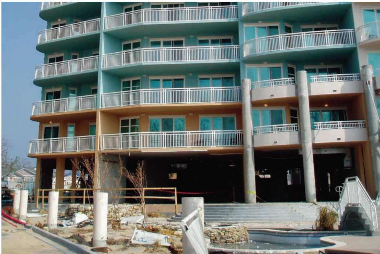
Figure 2-24 Condominium building in Gulfport, Mississippi, with wave and storm surge damage to non-structural elements at the ground floor, but no reported structural damage (FEMA 549, 2006).
